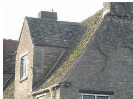
Repairs using traditional materials add to the aesthetic appeal of a property, as the new stone slates on the dormer at no. 42 show
