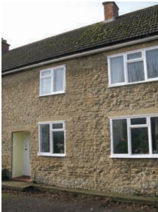
18 Crown Road - a possible join can be seen between the windows
